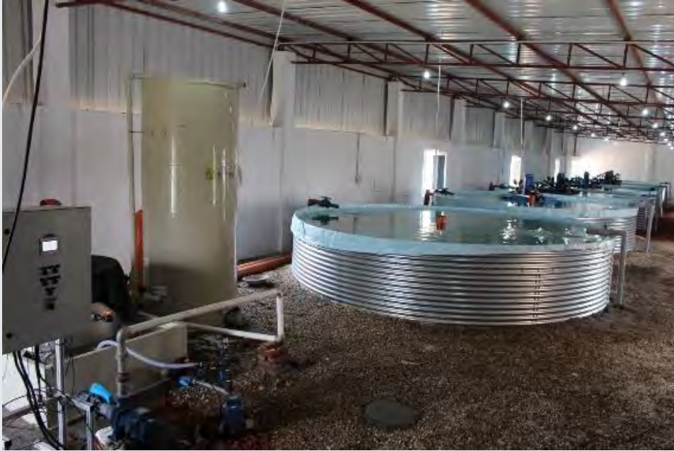
Turnkey Project North India – Barramundi
